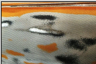
Rust forming under paint
